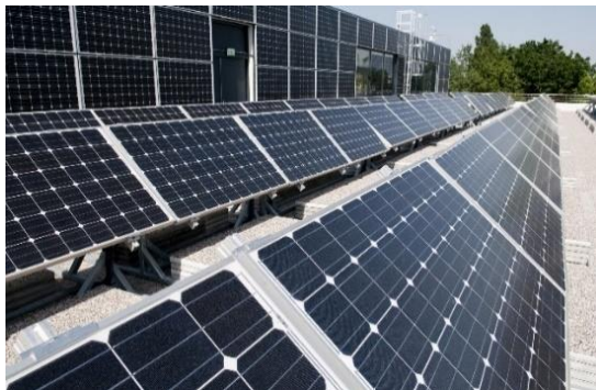
Fig. 1: PV array on the second floor of the experimental ADREAM BIPV in LAAS-CNRS.
