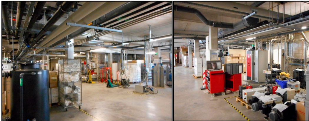
Figure 1. Industrial environments considered in this paper. The walls, metallic pipes and machines generate undesirable clutter that challenge the long-range detection and wireless reading of zero-power sensors for the monitoring of pressure.
