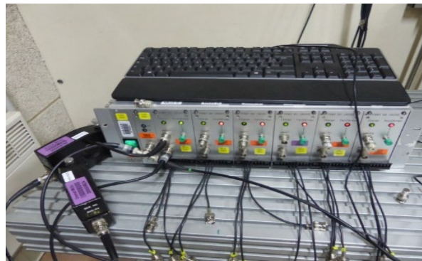
Figure 4. Somelec Wheatstone bridge and calibrated Rogowski coils on different cables.
