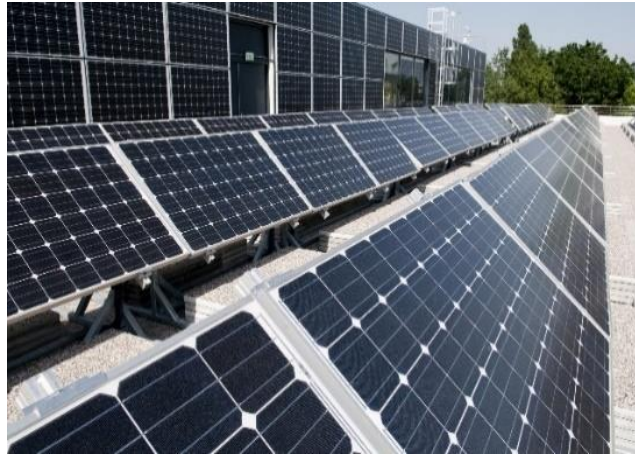
Figure 5.7 ADREAM building – Rooftop PV panels
