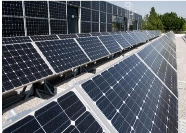
Figure 5.7 ADREAM building – Rooftop PV panels
