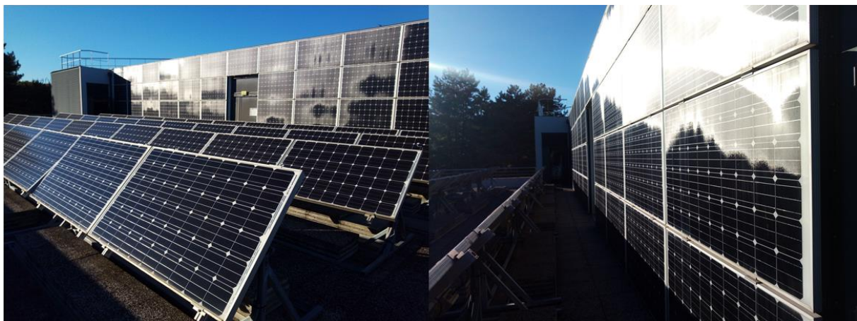
Figure 14: Regular crystalline silicon PV cells installed on the terrace and walls of the ADREAM building
