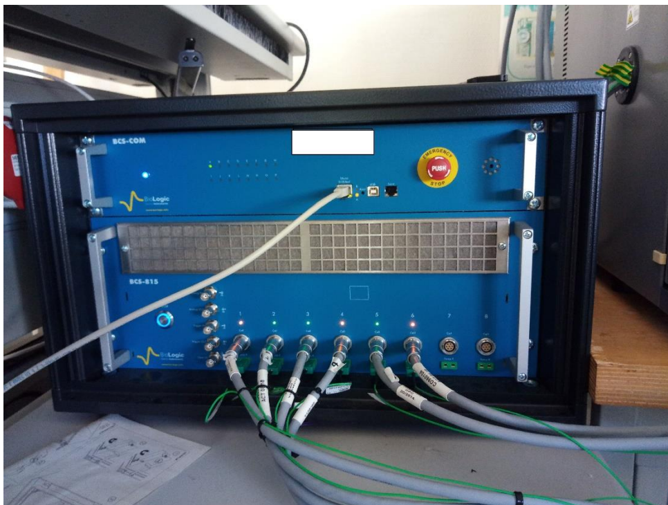
Figure 31: BCS-815 battery cycler from Bio-Logic installed in the laboratory room of the ADREAM platform
