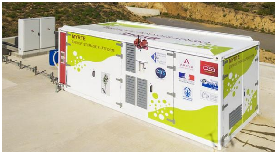
Figure 69: Electrolyser station for solar Hydrogen production of the MYRTE platform in Ajaccio
