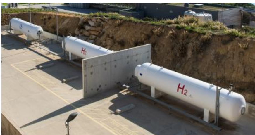
Figure 70: Hydrogen and Oxygen storage tanks at MYRTE platform in Ajaccio
