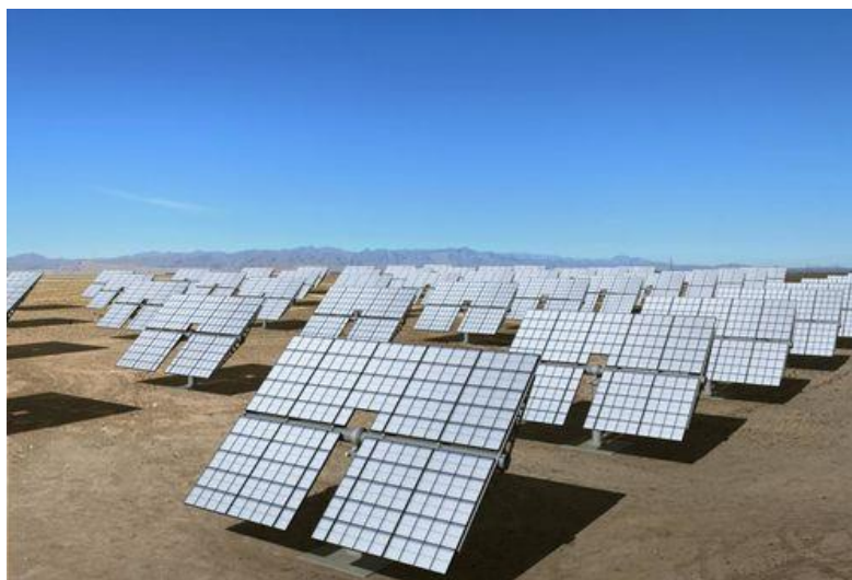
Figure 5: 1 MW CPV installation with trackers in Morocco, by SUMITOMO Electric
