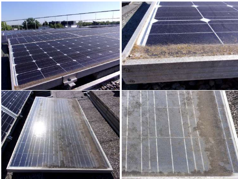
Figure 1.16 Example of dust accumulation on a PV module
