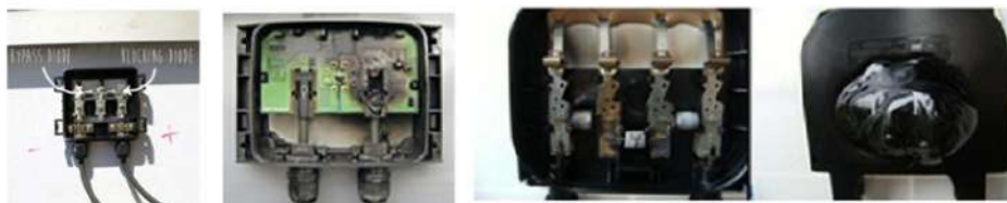
Figure 1.21 Failure of diodes in PV modules [54]
