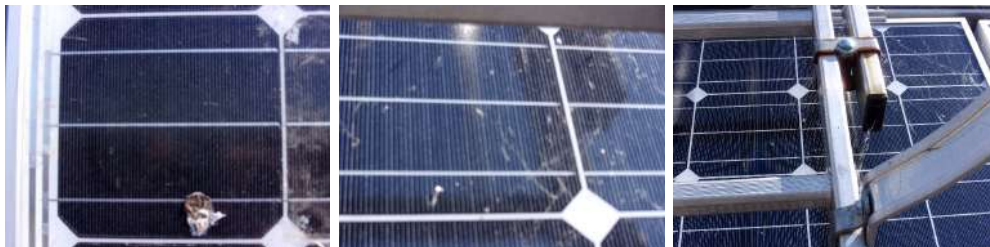
Figure 1.17 Example of other types of obstacles generating shadow problems on PV modules (bird droppings, cobwebs, and fixed obstacles such as stairs)
