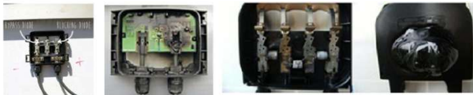
Figure 1.21 Failure of diodes in PV modules [54]
