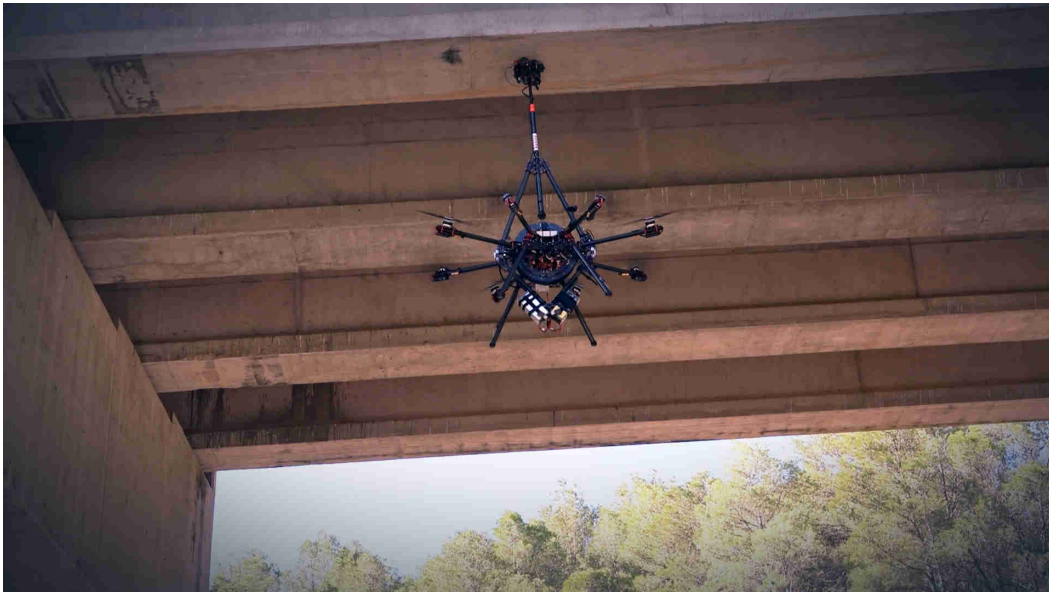
Figure 11.12 – The AeroX platform performing the contact inspection of the underside of a bridge.
